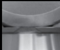
Fractured inner ring rib
