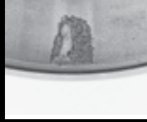
Resulting localized spalling in raceway
