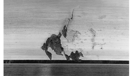
Fig. 1: Point Surface Origin (PSO) spalling
