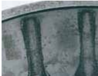
Staining: Surface stain with no significant corrosion from moisture.
