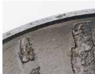
Line spalling: Roller spaced spalling from bearings operating after etching damage.
