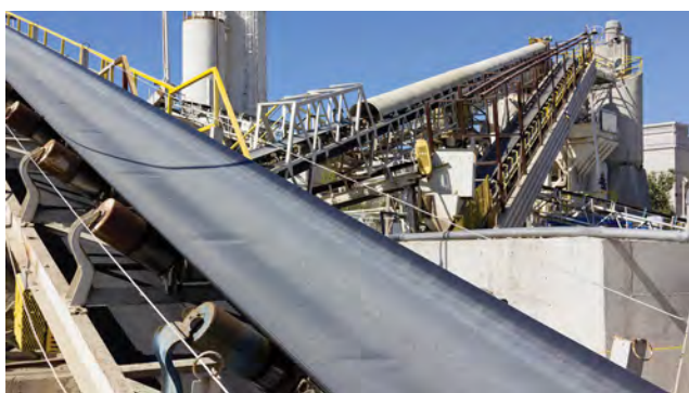
Figure 4. There is often only a small window of opportunity to lubricate bearings in critical equipment without disrupting operations.
