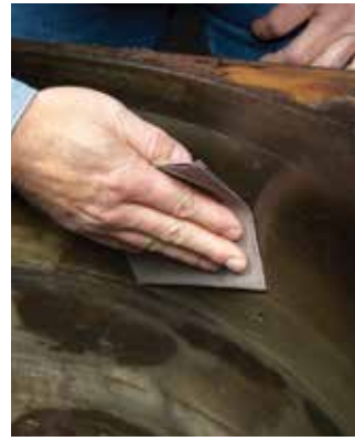
Fig. 23 Remove any heavy corrosion or fretting in the chock
