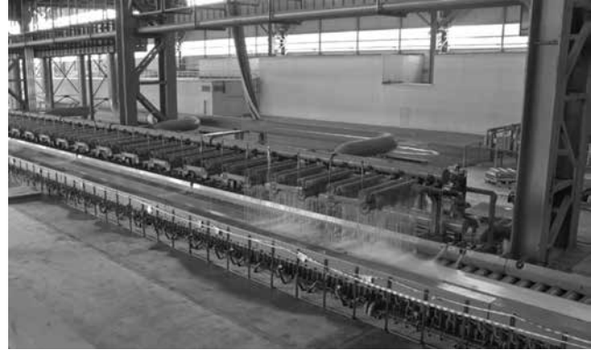
Fig. 110. Hot-strip mill roller tables.
