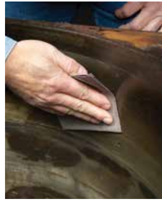
Fig. 23 Remove any heavy corrosion and fretting in the chock
