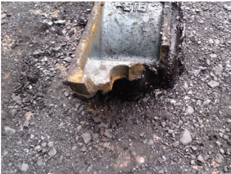
Figure 4: Broken baseplate of a cast-iron pedestal bearing.
