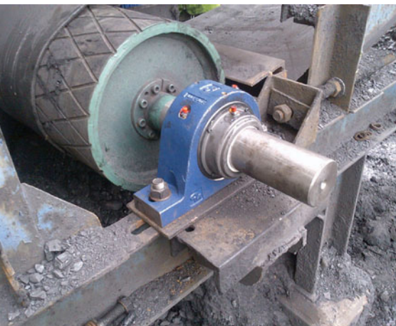
Figure 2: A spherical roller bearing solid-block housed unit installed on a conveyor at a coal mine.
