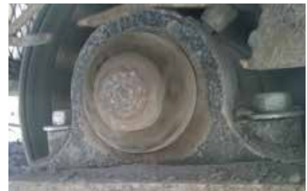
Conveyors at Boxley's aggregate quarry mill now run on Timken Type E tapered roller bearing housed units, resulting in greater uptime and reliability.
