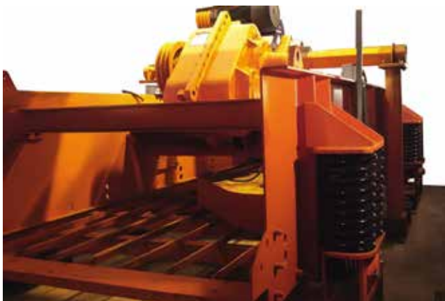
Fig. 21a Coal crusher shaft
